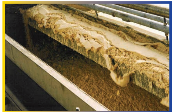
View of separated material from DAF unit.
